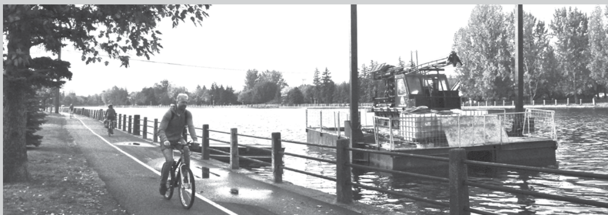
Crews began drilling in the Rideau Canal at the beginning of October, preparing for construction of the Mid-town footbridge.
