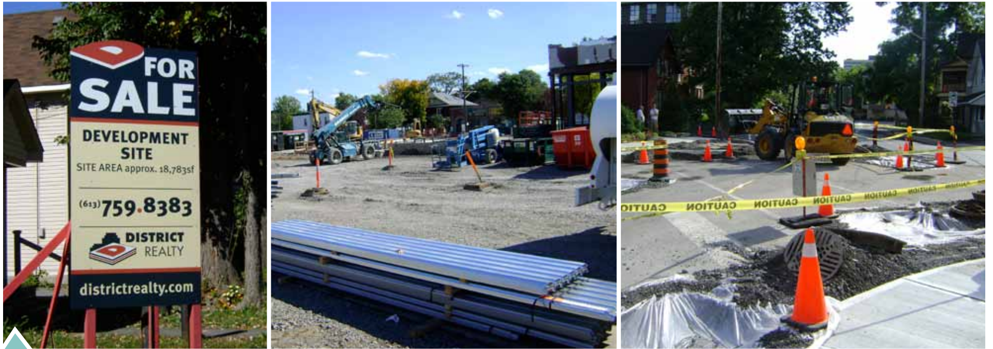
The north end of Old Ottawa East seems to be on track for extensive development. Between the boundaries of Harvey, Concord, Greenfield and Main, there are three areas which have been sold for development: a duplex on Harvey, a triangular section including two houses on Concord between Montcalm and Greenfield, and the former Legion at 99 Greenfield. So far, work has only been done on the Concord/Montcalm/Greenfield property. Then, in mid-summer, a sign went up on the triangular property at the Havelock/Greenfield split.
