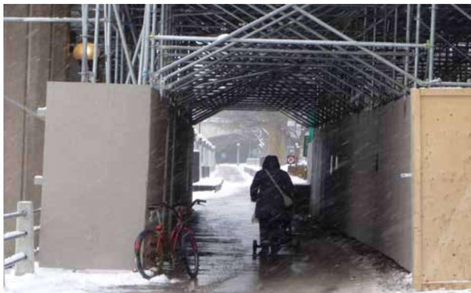
The NCC ensured that there would be a continuous pathway connection during the rehabilitation of the Mackenzie King Bridge and this may also be required when MTO replaces the 417 Canal bridge.
